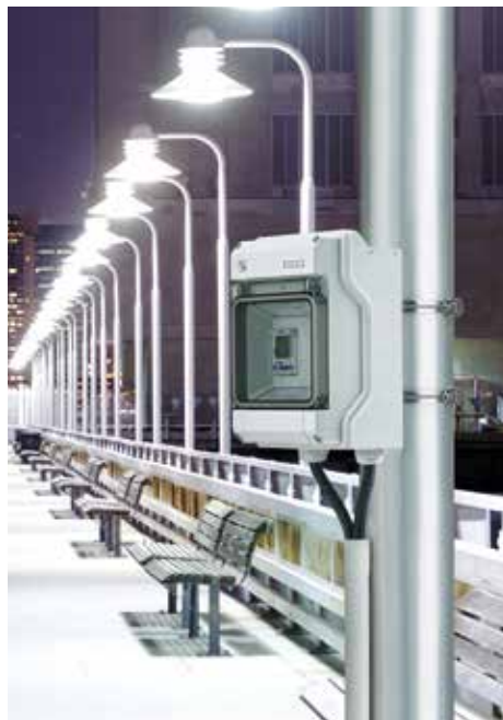
Pole mounting of KV small-type distribution boards
