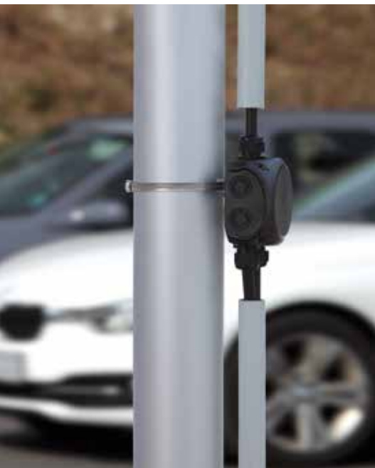
Pole mounting of cable junction boxes
