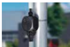
Power supply of a security camera in public area
