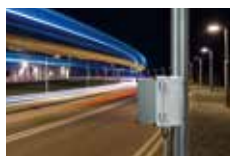
Street lighting control
